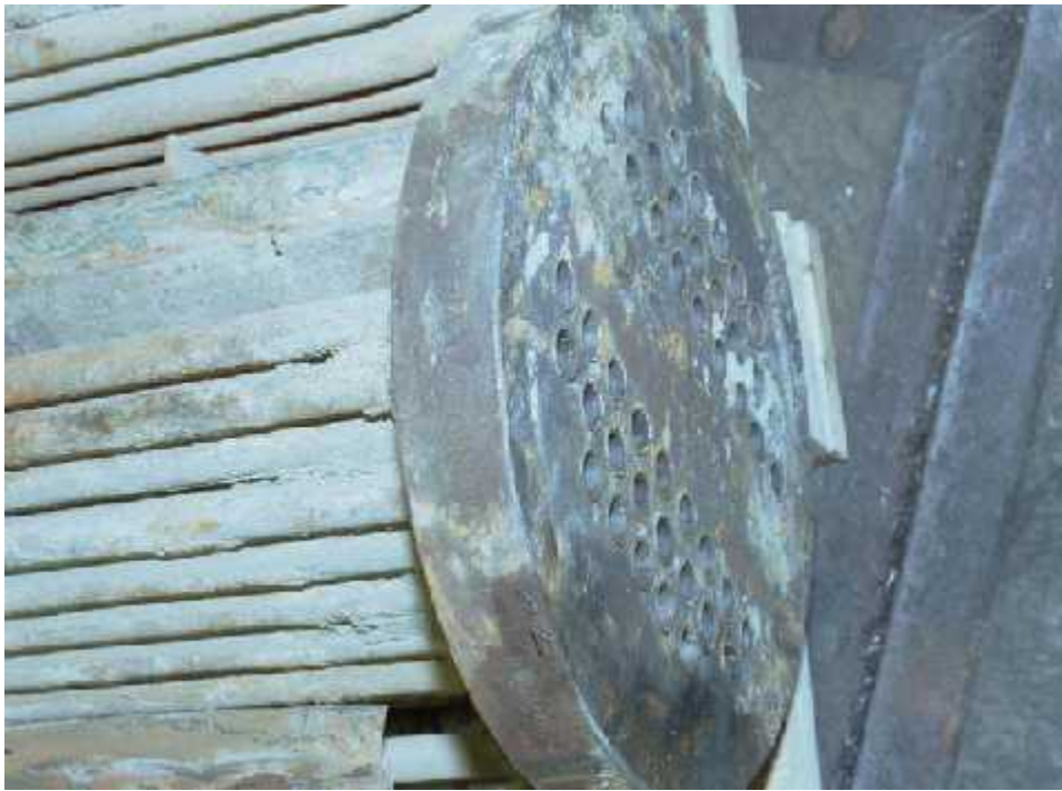
Process water inside tubes 180 °C Cooling water outside tubes ambient temperature Scaling after six months without SW
