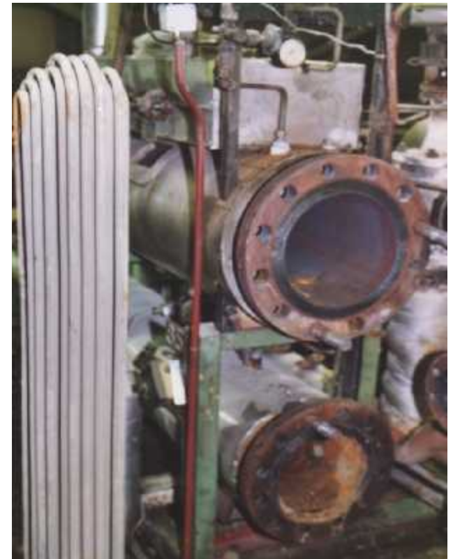
Completely clean after being treated with SW during six months
